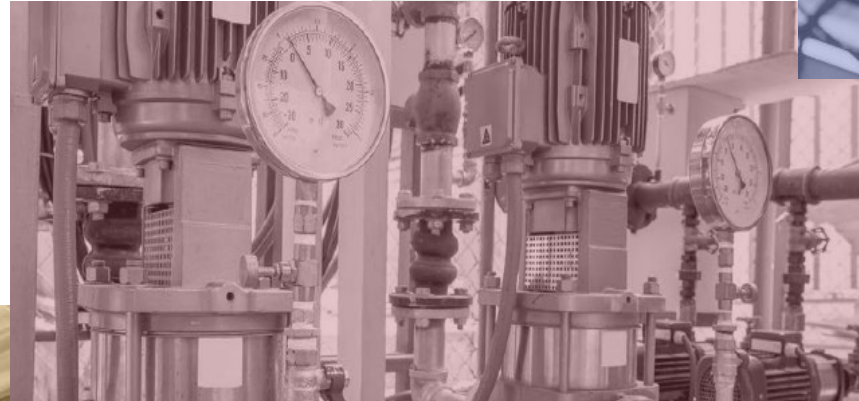
Pump System Optimization
