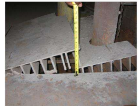
Top: hole in hydrogen pipe Bottom: cover plates dislodged by explosion
